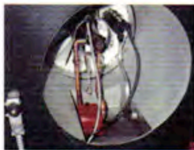
MonoMag installed on incoming fuel line
