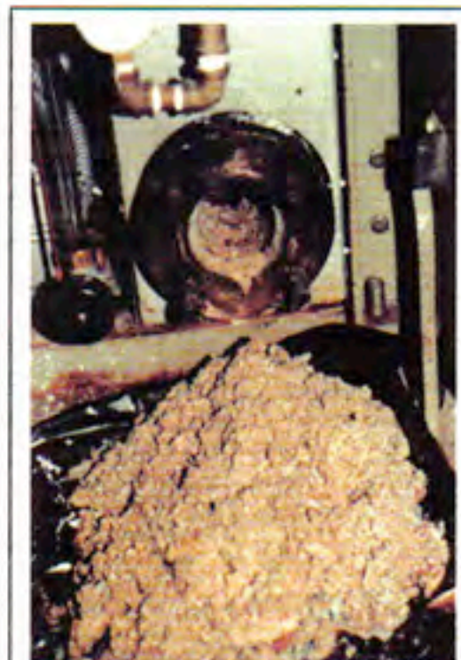
Hard scale easily removed as a soft slush after MonoMag water treatment
